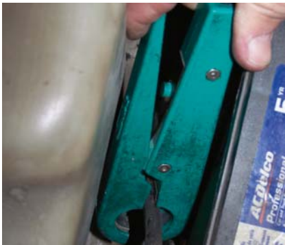
P12-4 Connect the inductive pick-up around all battery ground cables.
